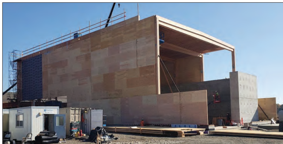
Oregon State University's A.A. “Red” Emmerson Advanced Wood Products Laboratory under construction in fall 2018. Mass-plywood panels (MPPs) manufactured by Freres Lumber Co. in Lyons, Oregon, were used to build interior and exterior walls. Image: OSU.
